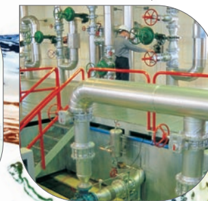
<< Industrial Process Systems
